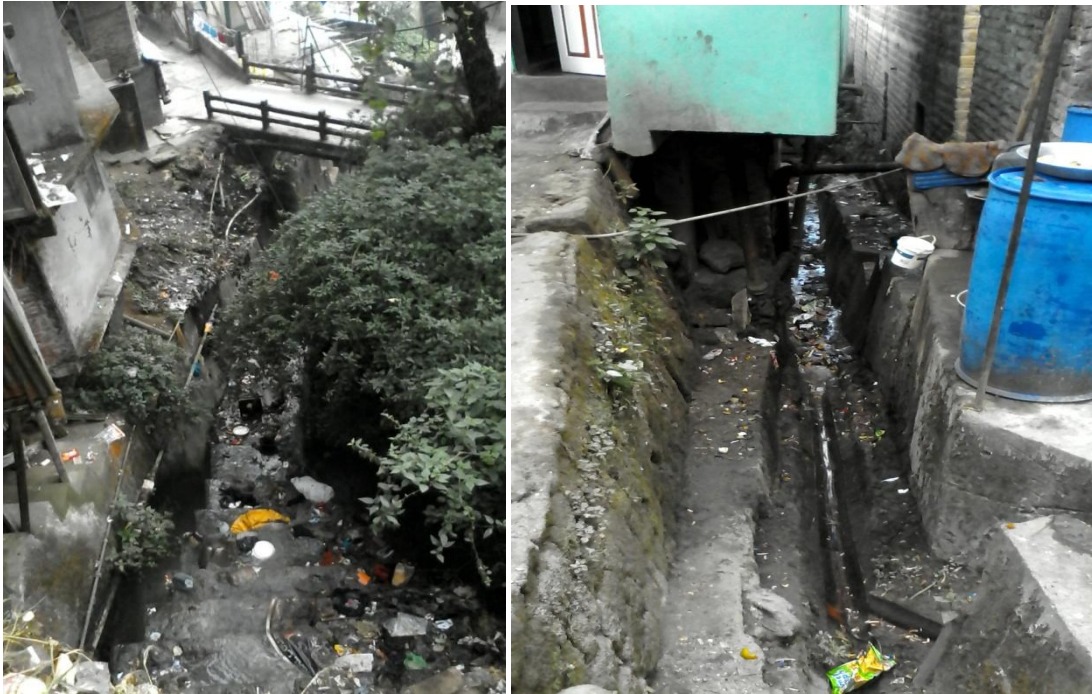
Figure 4.7 Sewage and Drain
