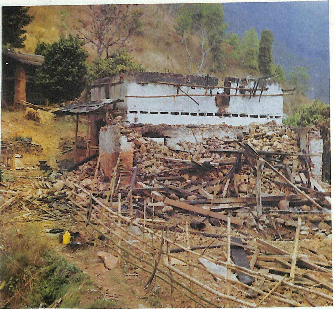
Two houses burnt down by terrorists. A gang of 20 terrorists raided three houses in Harabotey village in Chirang district on 16 April 1993. Two of the houses which belonged to Kharka Bahadur Dahal was burnt down by the terrorists after being ransacked.
