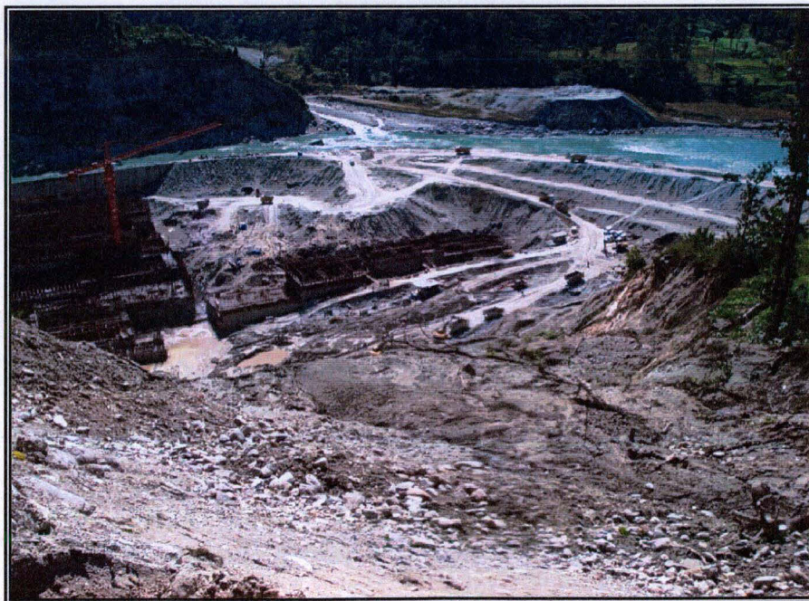
Plate 4.5: Dynamics of Development NH31A that run-along a little above the construction site of Teesta Hydrel Dam [Stage III] was washed down during the monsoon of 2006 [Photo: Vimal Khawas, October 2006]
