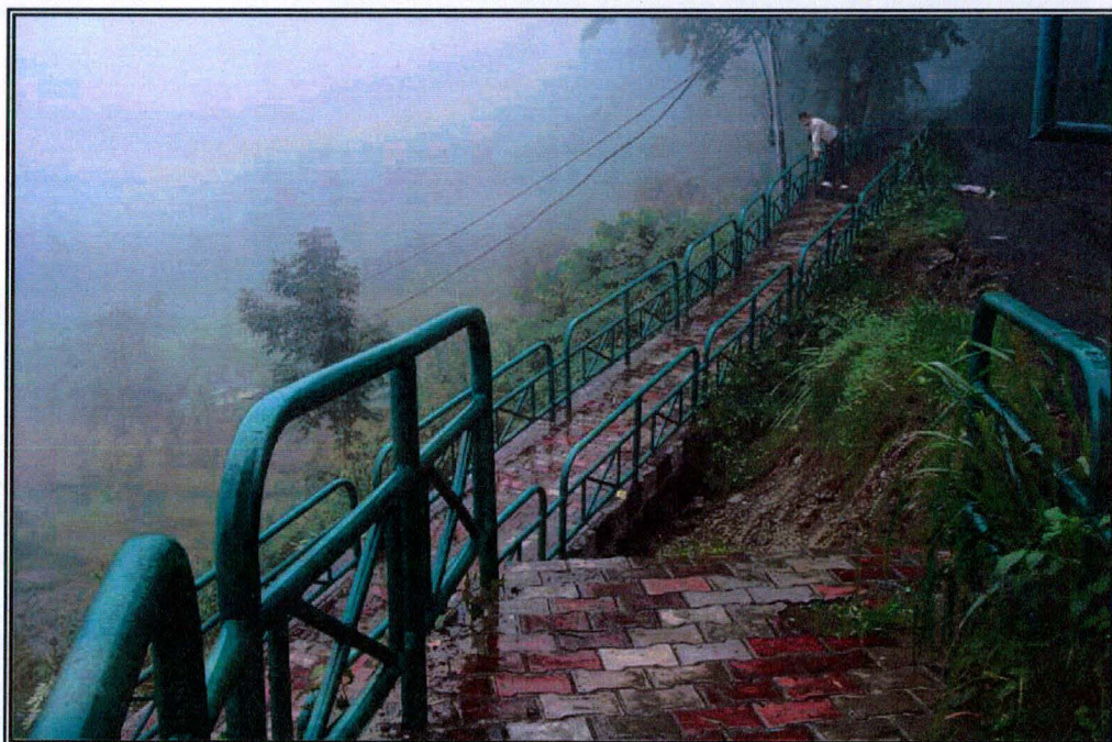
Plate 5.3: Mudslide destroys Footpath in South Sikkim
