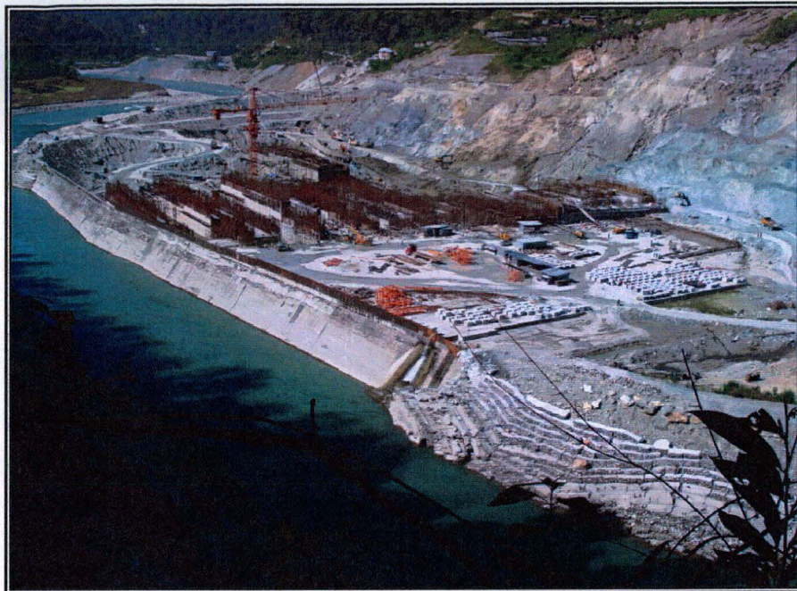
Plate 4.4: Taming River Teesta Teesta Hydrel Project Stage III under construction. [Photo: Vimal Khawas, October 2006]
