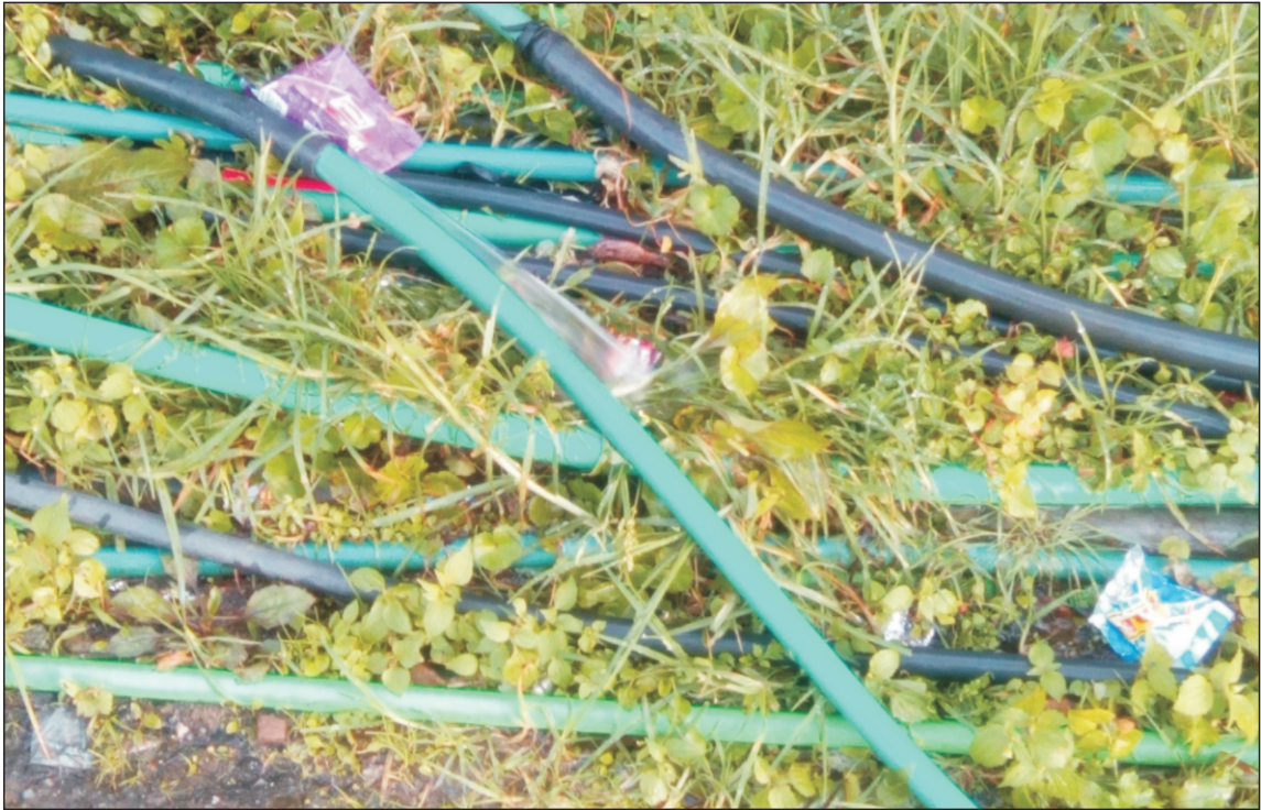
Plate 8: Water Leakage from Pipe
