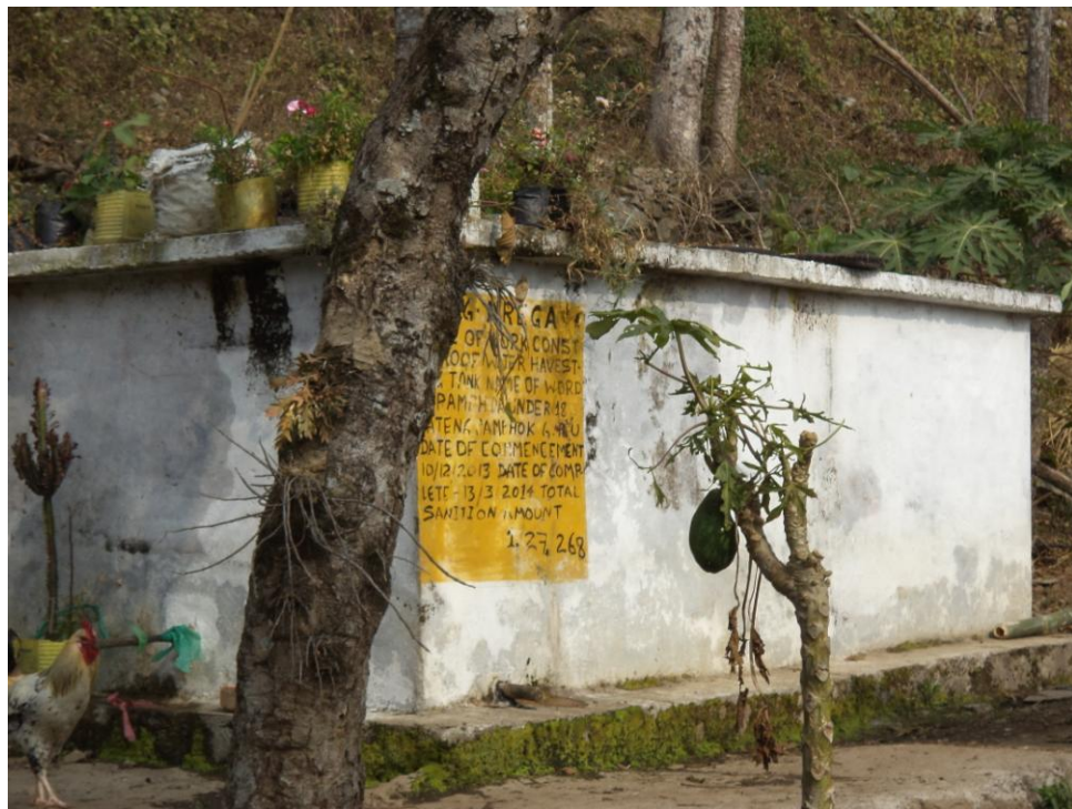
PLATE 3.11: Water harvesting tank provided by MGNREGA in Mellidara (Photo- Rashmita Sarkar, July, 2016)
