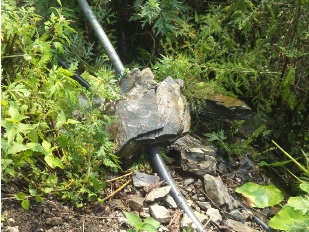
PLATE 4.5: Pipe connectivity from source (Khani Khola) to the village (Photo- Rashmita Sarkar, April, 2016)
