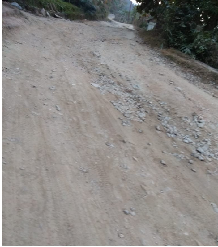
Fig 4.1.1 Condition of road leading to Tinchuley (Source- Field Survey- September, 2018)
